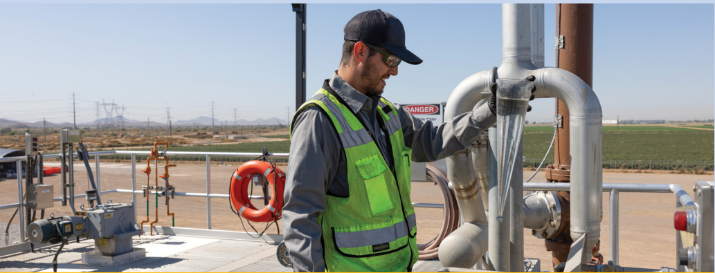
Surface Water Facility operator inspects the sand ballast system, a key part of the water treatment process.
