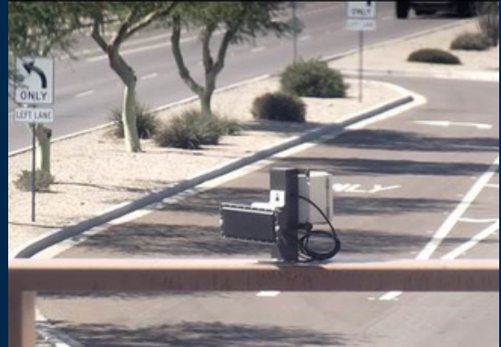
A photo of the radar detection equipment. These devices are installed throughout the city, either mounted on top of modular (rectangular) signal arms or attached to round ADOT-style signal arms.
