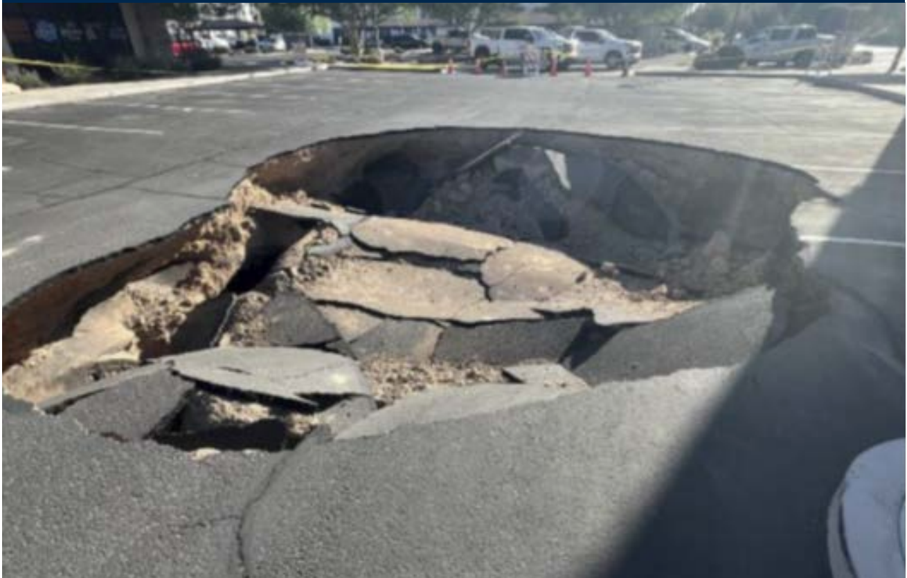
ORIGINAL SINKHOLE - OCTOBER 2025
